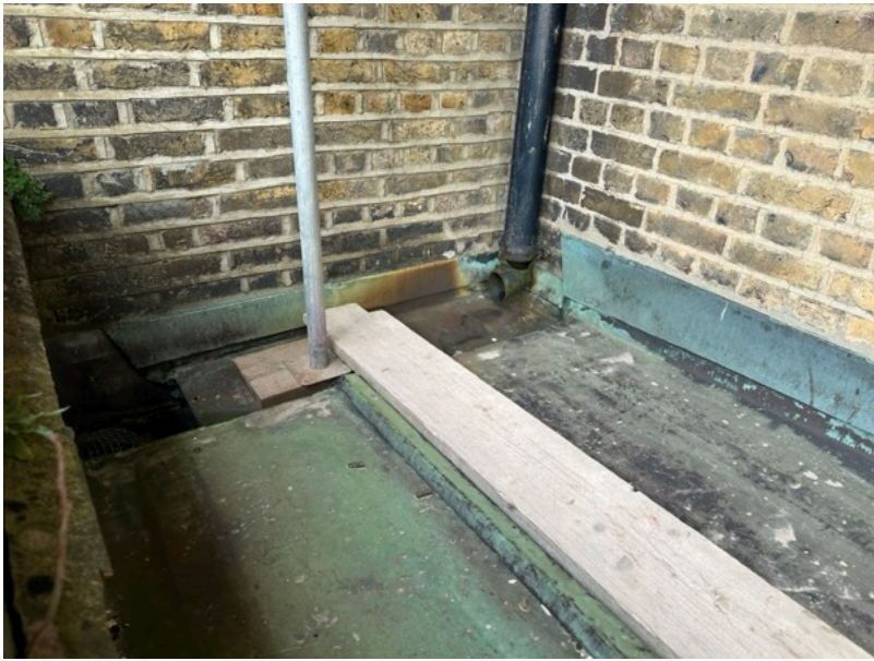
Photo 23 Location: Church (West Elevation) Replace damaged shoe to rainwater downpipe.
