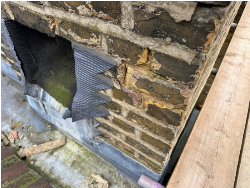
Photo 14 Location: Church (East Elevation) Repoint all eroded and missing mortar pointing around the hopper outlet to the tower roof.
