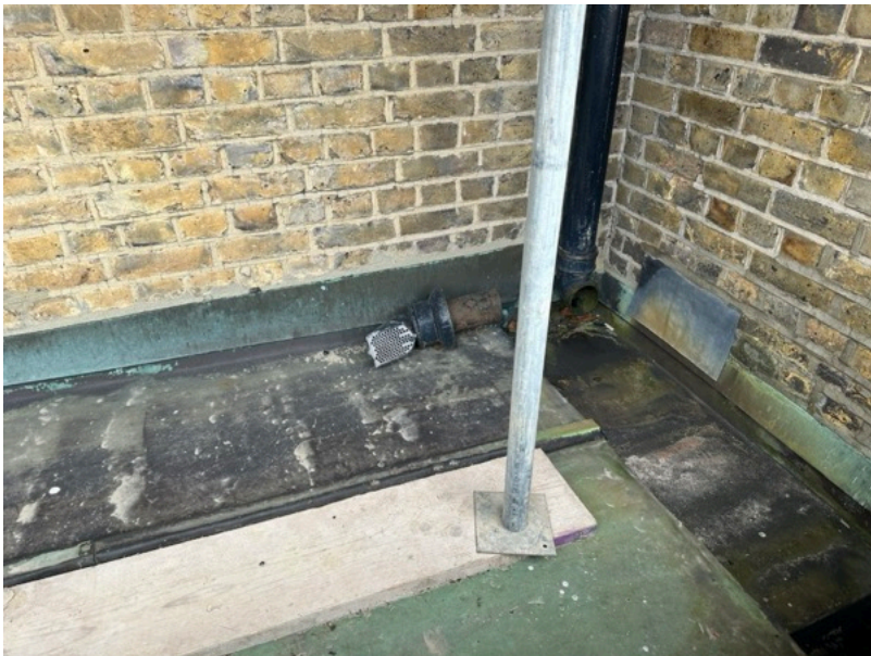
Photo 24 Location: Church (West Elevation) Reuse redundant shoe to fix downpipe in photo 23
