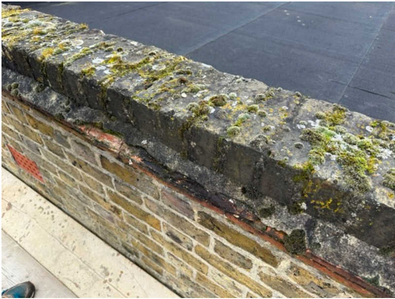
Photo 13 Location: Church (East Elevation) Comment as per photo 12.
